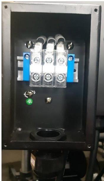
Figure 11: Electrical Connection Box
