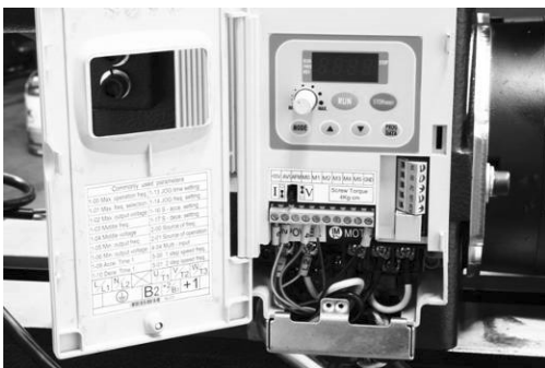
VFD with cover open
