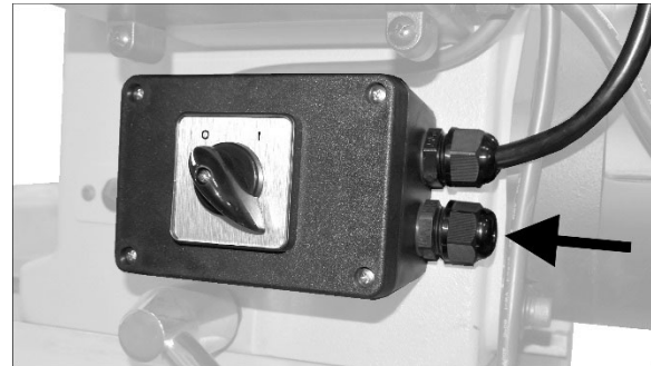
Figure 7-1: main switch box
